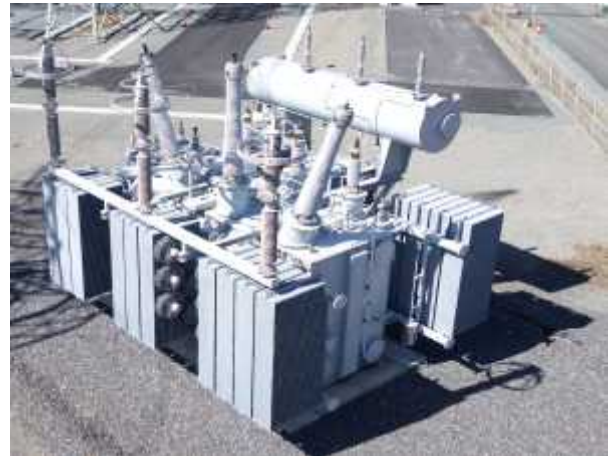
POWER LINE - HIGH VOLTAGE SUB-STATION
